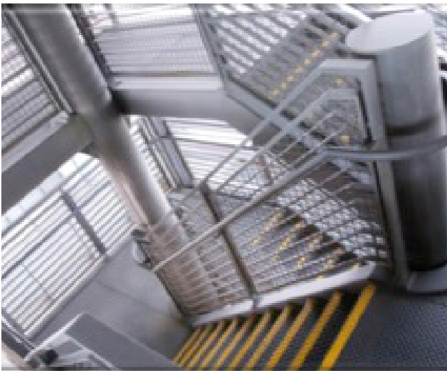
A steel staircase with colour-contrasted nosings provides an example of good stair design. The design would have been even more accessible for people with vision loss if colour contrast had been applied to the handrails.
