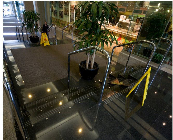
An example of poor stair design – black stairs with no colour contrast on the nosing.
